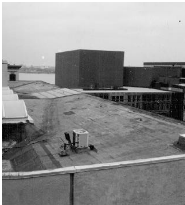
Rooftops should not be magnets for mechanical or communications clutter that can disrupt public views. Consider views from the street when positioning such equipment.
