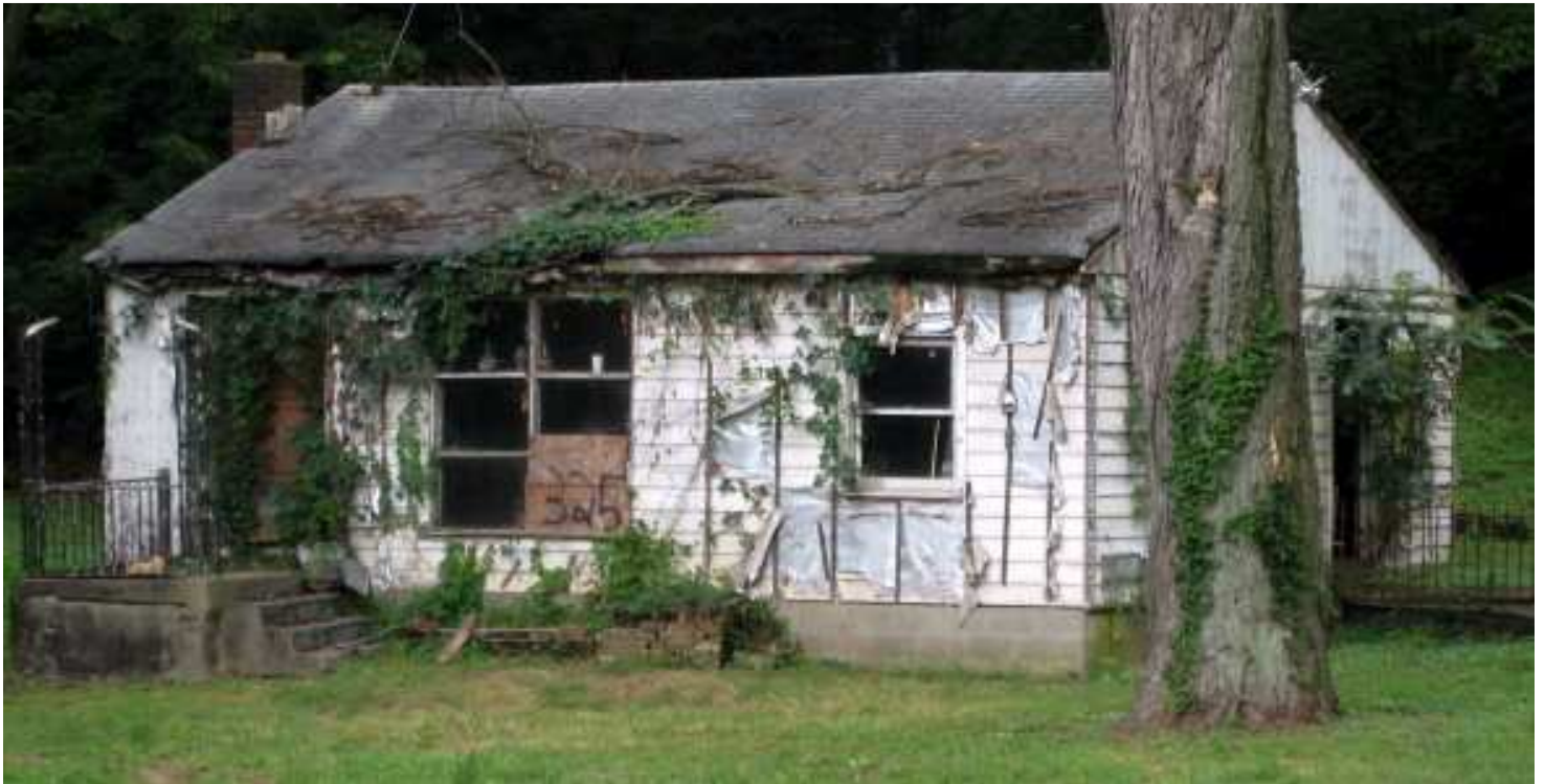
Demolition by Neglect is against the law – the Metro property maintenance code.
